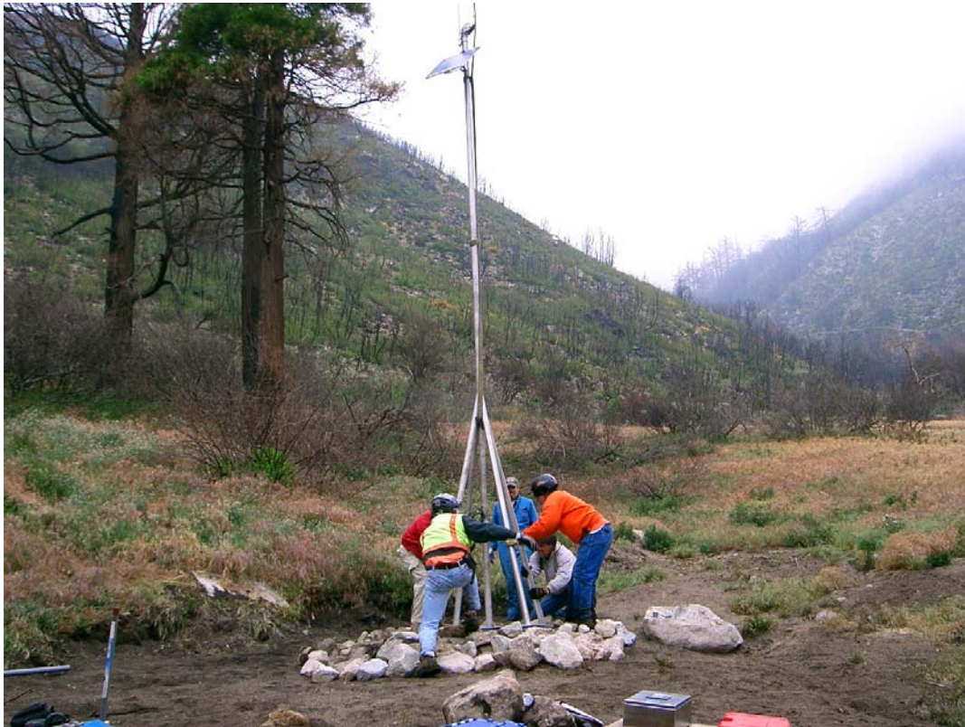
INSTALLING SOLAR PANEL AND ANTENNA MAST AT ONE OF THE SPRING SITES
